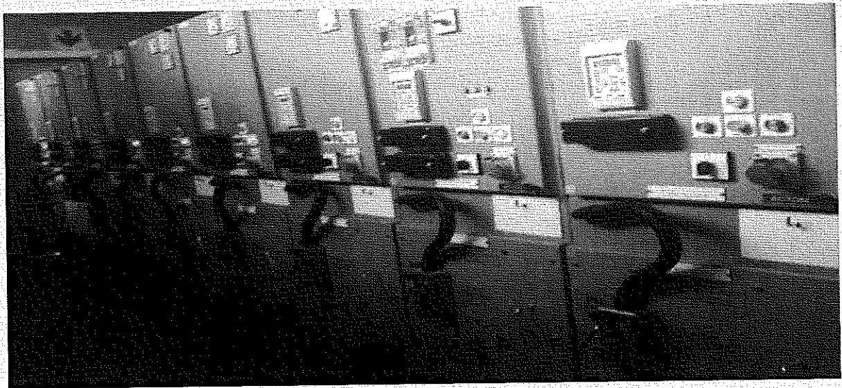
FIGURE:4 BELA-BELA SUB STATION
