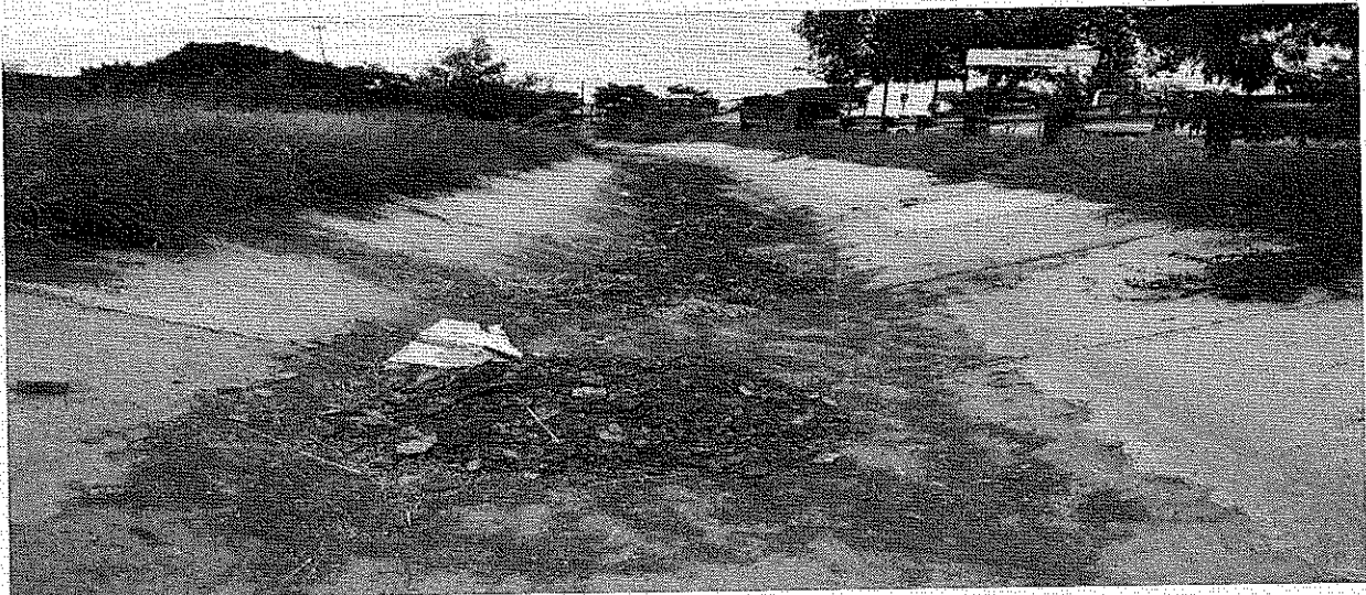
Dirty Stormwater Drainage System
